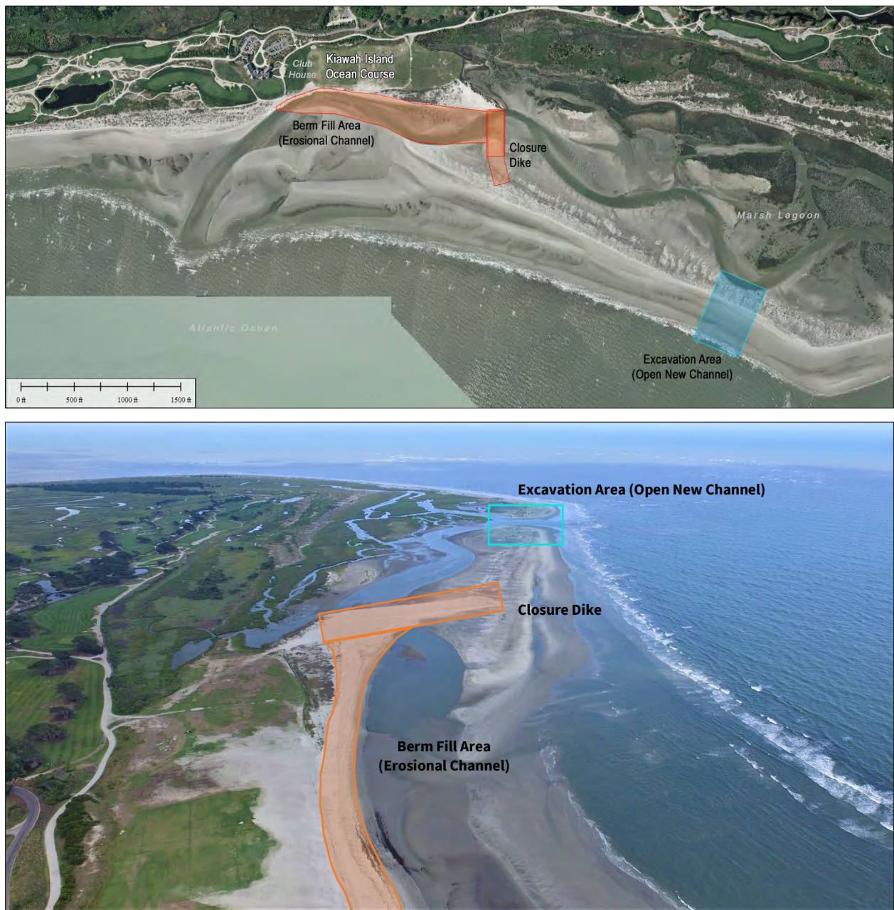
FIGURE 2.10. [UPPER] Excavation and fill areas used in the 2015 project. Approximately 100,000 cy of sand was transferred from the excavation area to the fill. [LOWER] Project area on 7 July 2015, after project completion, showing closure dike in the center of the image and a new flushing channel at the upper right. Encroachment by the ‘erosional channel’ destroyed hundreds of feet of dunes, leaving no protection in front of the driving range.
